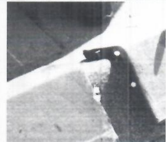
Fig. 3a. V Ridge Tiles with three (3) ring shank nails adjacent to the tail
