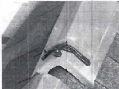
Fig. 1b. Two 6-in. long 0.25-in. wide beads of MasterSeal NP 1 at fastened tail of Lap Ridge Tile
